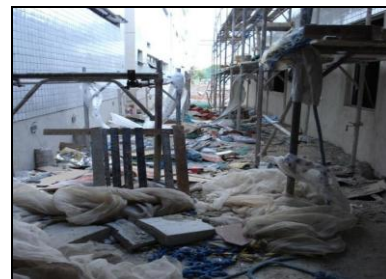
Fig 2: Inadequate provision of RCCD in a public work. Source: the authors.
