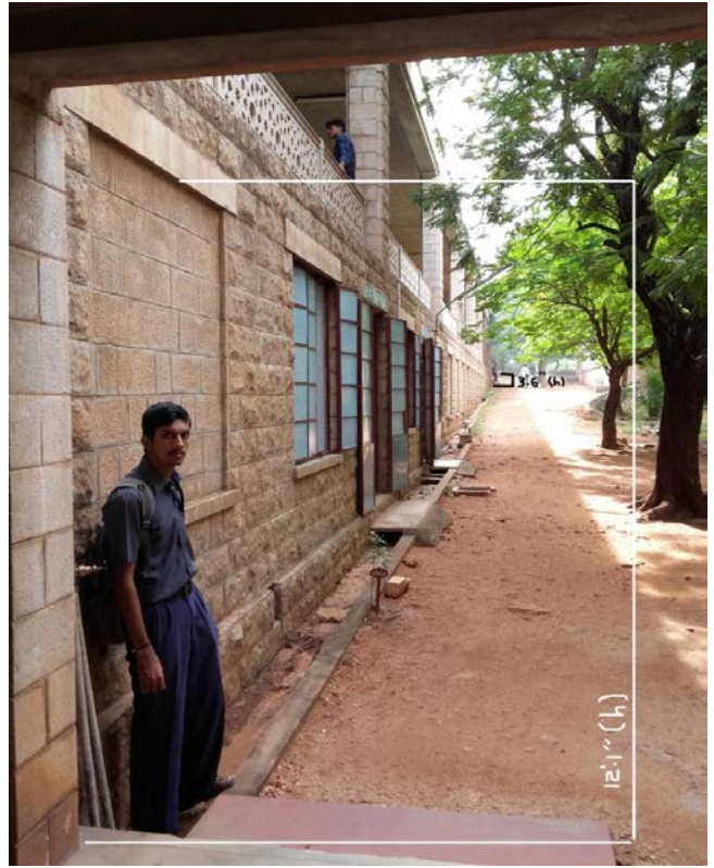
Fig 7: The Mechanical Department shows the block's slope-nature (If you zoom this picture the other end again palced with a boy to show how that end is very shorter).
