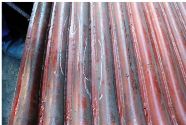
Fig 10: Shows Butt joints of fin are not ground flushed
