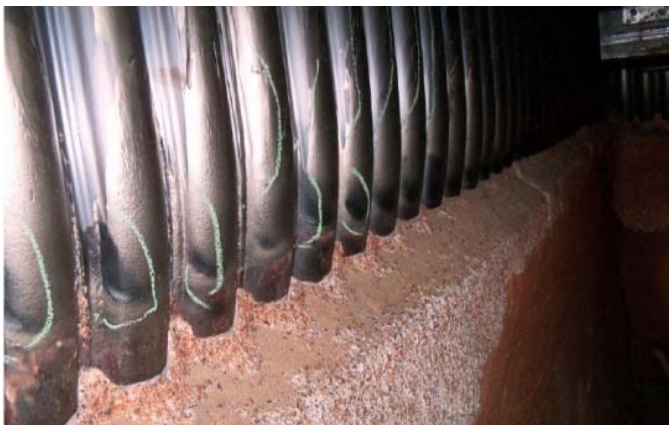
Fig 1: Shows erosion found in kick off zone
