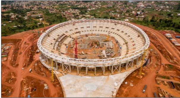
Fig 4: A 2018 image of the Paul Biya stadium under construction on the site where the Yanda community says their ancestors are buried. Image by Nana Padrino via Wikimedia Commons (CC BY-SA 4.0).
