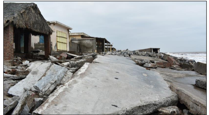
Fig 3: Thinh Long Beach resort has appeared 4 places of landslides and collapses on the sea embankment and the surrounding area
