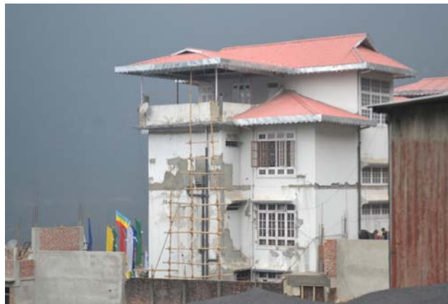
Fig 2: Severe damage building under repair
