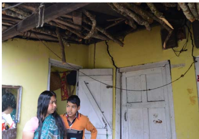
Fig 5: Kuccha house with severe damage
