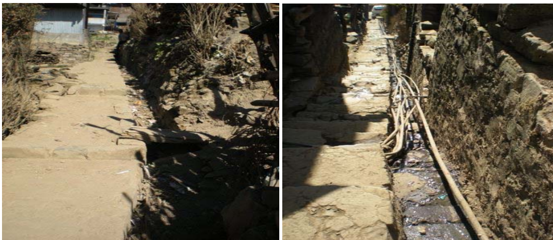
Plate 3: Poorly maintained drainage system in the Area (Pfutsero Town, Nagaland)
