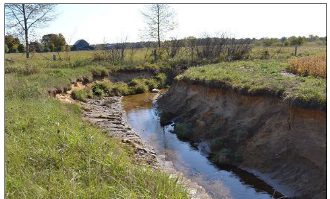
Fig 6: Bank erosion involves the undercutting and scouring of natural stream and drainage channel banks.
