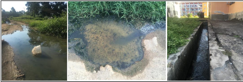
Fig 2: Formation of sewage pond Grey water in Uncovered drains
